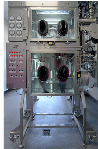
Module 9 (2nd floor) Filter dryer isolator
